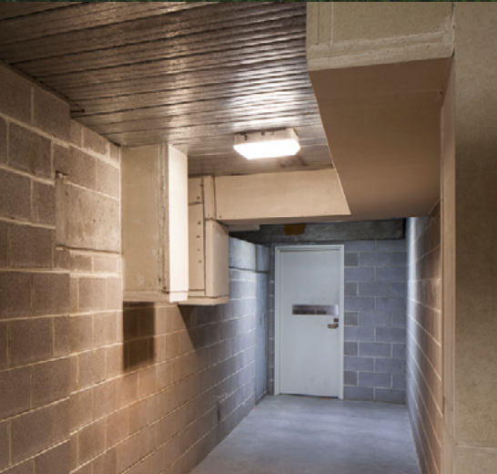
Fire stair corridor chamaeleon lights
