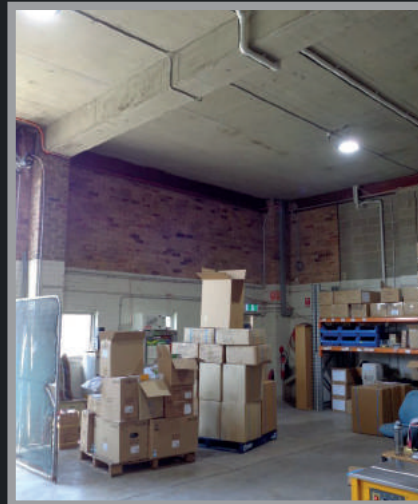
150W Stargate in warehouse entry
