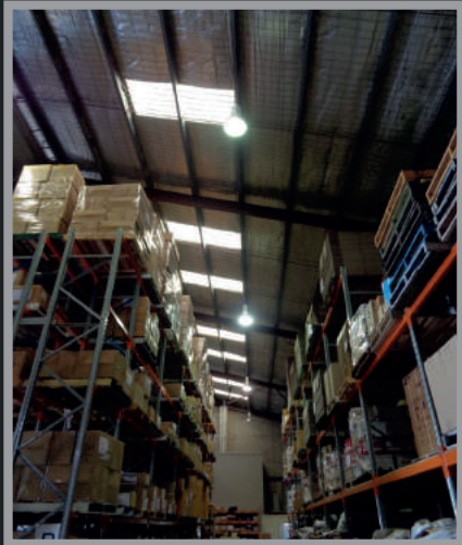
Existing 400W metal halide fittings
