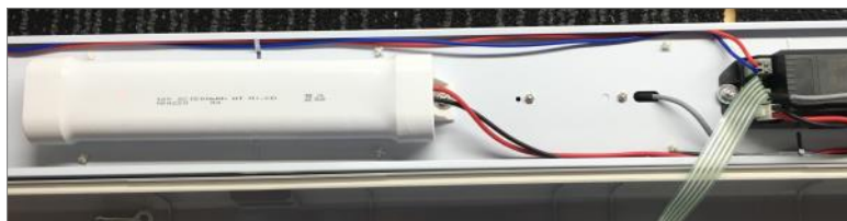
The battery is screwed to the gear tray.
